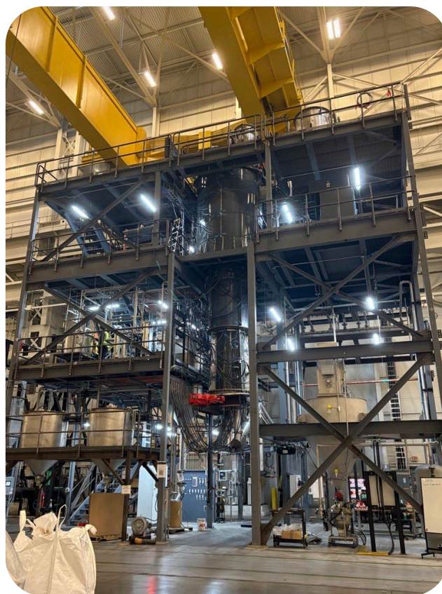
Figure 1 Mass Production Furnace at Riverside Facility in Chattanooga, Tennessee.
