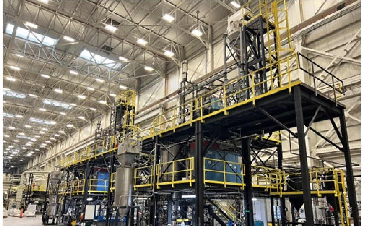
NOVONIX Generation 3 Continuous Induction Furnace Systems, Chattanooga, TN
