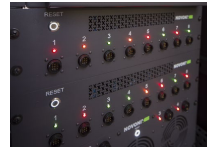
Diagnostic tools and performance testing
