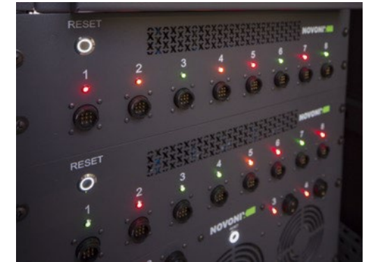
Diagnostic tools and performance testing
