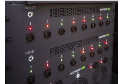
Diagnostic tools and performance testing
