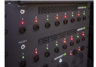
Diagnostic tools and performance testing
