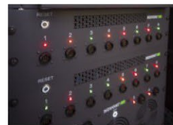
Diagnostic tools and performance testing
