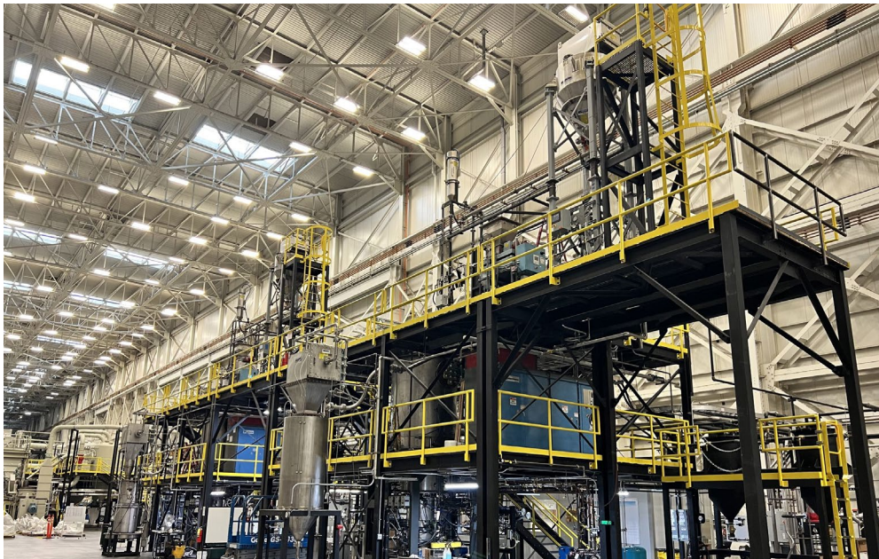
Two Generation 3 Furnace systems and milling equipment installed in NOVONIX's Riverside facility
