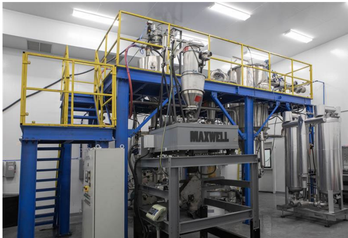
Cathode Pilot Line with nameplate capacity of 10 tpa
