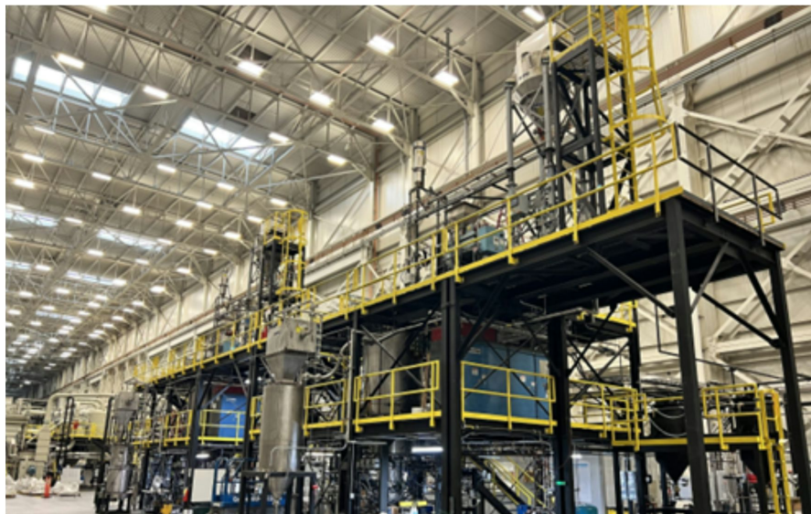
NOVONIX Generation 3 Continuous Induction Furnace Systems, Chattanooga, TN
