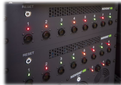
Diagnostic tools and performance testing
